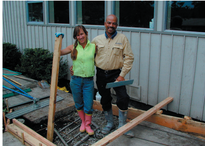
Rita Baxter and Alvin Johns frame the new ramp at the Unity entrance. Thank you for the great work!
